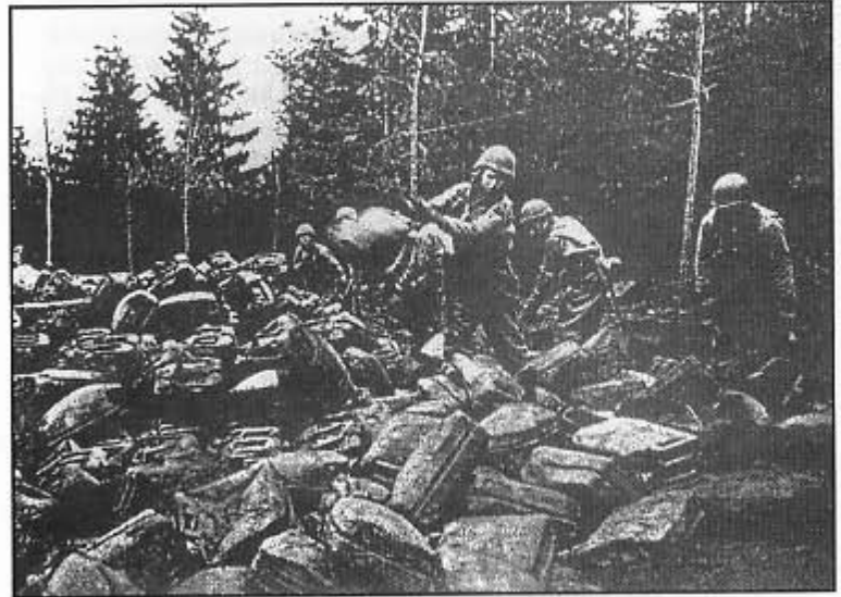
Demolition in progress on the Francorchamps Road above Stavelot. Pictured left to right: Sgt. Bob Hyde, PFC Willie Esparza, PFC Bill Shureck, PFC Clifford Rutledge; Forefront Edward Richardson, PFC Joseph Stec, all of the 526th Armored Infantry Battalion, Company A.
